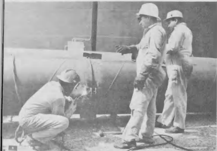
Welder M. Roga (left) and Boilermakers B. Kelly (c) and C. Bernabela do their share of the work.
